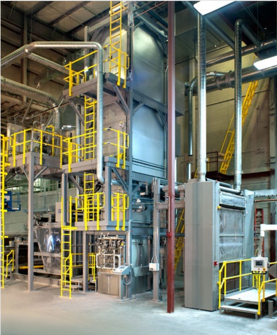
Two Sided Coater With Tower Dryer
