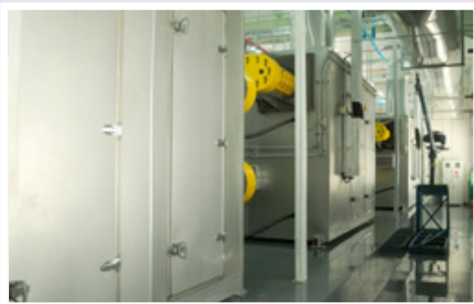
Installed Dryer Apparatus Units
